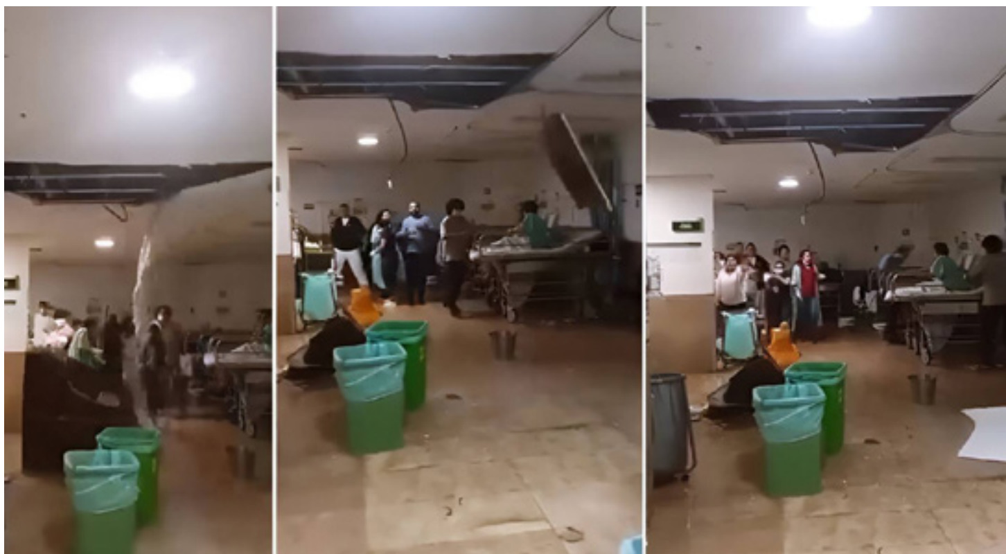
Image: "Ceiling of IMSS in Cancun collapsed" at https://www.elimparcial.com/mexico/2024/03/25/colapsa-techo-en-imss-cancun-en-sala-de-urgencias-cual-fue-la-causa/
